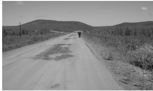
Fig. 6. Frost pumping of JDH.
