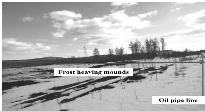
Fig. 4. Frost heaving mounds around the oil pipeline.
