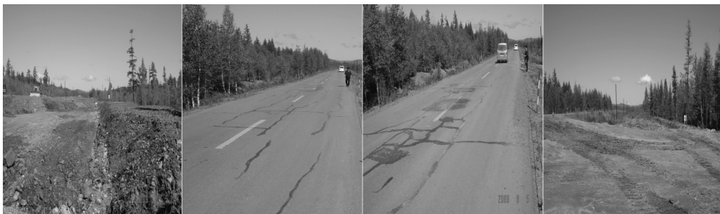
Fig. 5. Longitudinal cracks of JDH.
