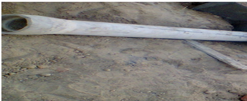
Figure 4. Pipe for Digestate
