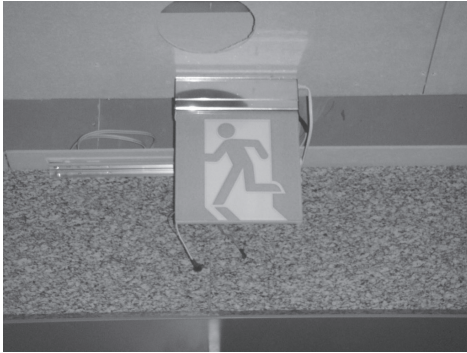
Fig. 3. C.P. Exit (not actuated)
