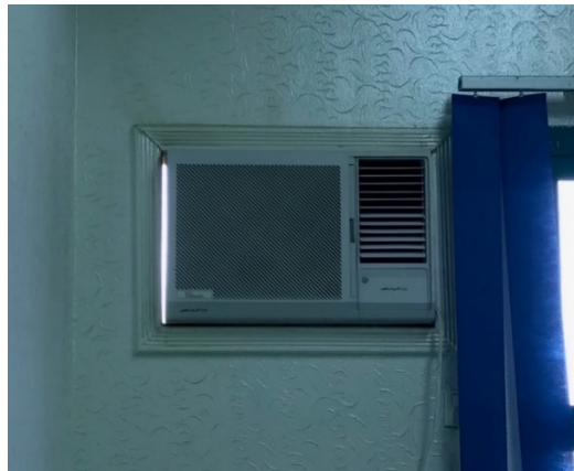
Figure 2. Infiltration gap in perimeter wall where the window-type AC is installed.
