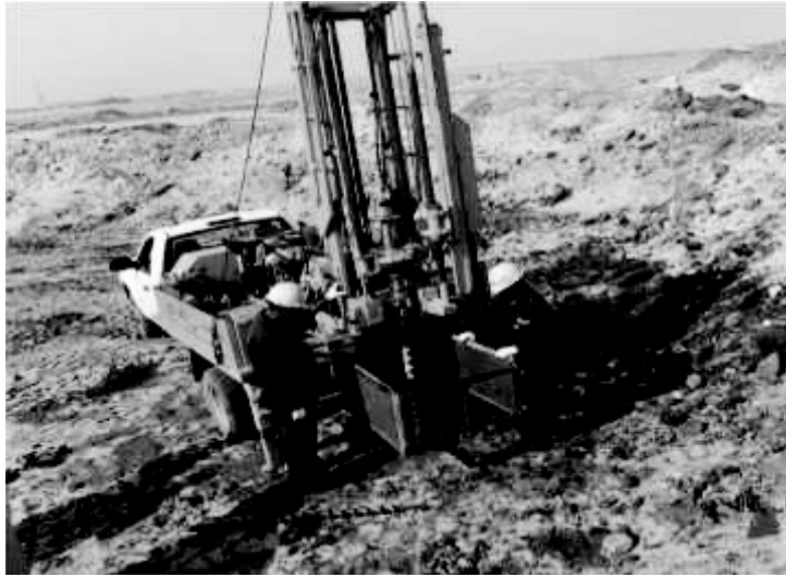
Figure 4. Soil sampling process using auger boreholes drilling techniques at the tested area.
