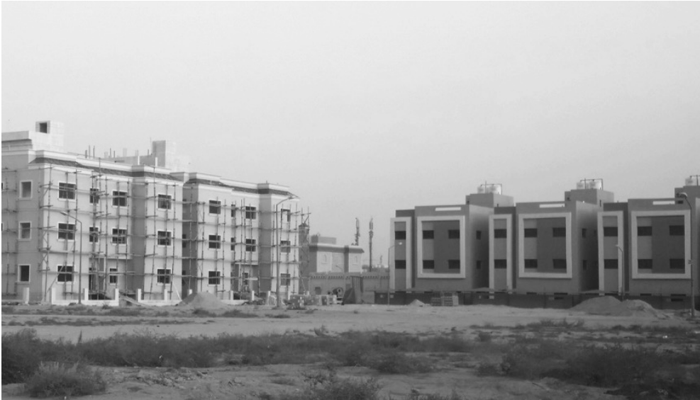
Fig. 9. This image shows commercial apartment buildings being built in new residential areas of AlSidiq. Source: The Author, 2015.
